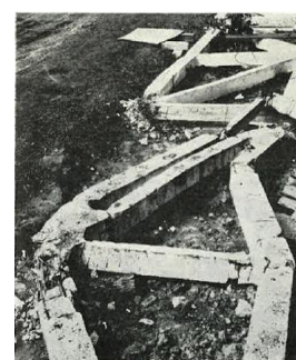
Fig. 3 Truss girder collapse in the Czechoslovakia from 1960s [5].
