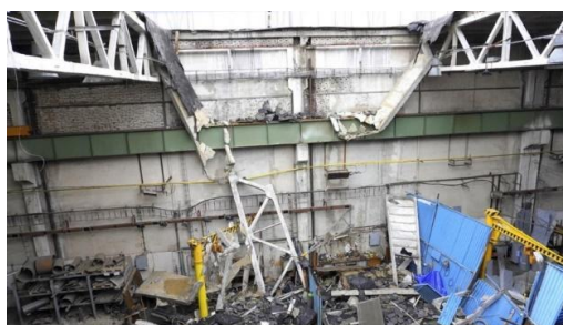
Fig. 2 Truss girder collapse in the Czech Republic from 2023 [4].
