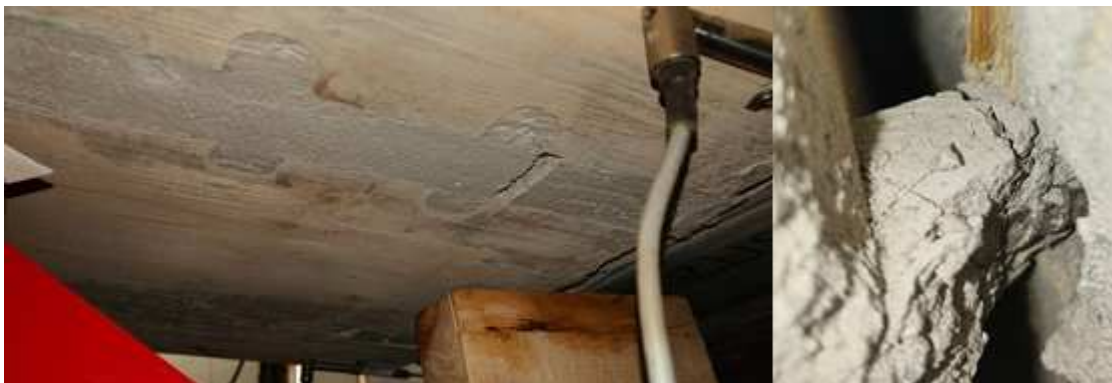
Fig. 52 Failure modes in specimen: cracking of concrete, fell out concrete, disclosure of rod.
