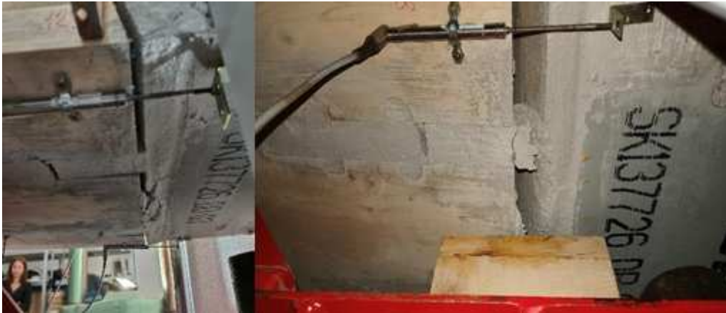
Fig. 41 Crack pattern development in groove.
